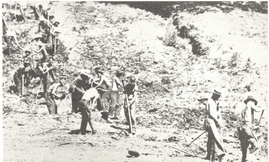
First work on the hatchery began in 1940 as a WPA project. The hatchery site was cleared, pond drains built and one residence completed before construction was halted by the outbreak of World War II.
